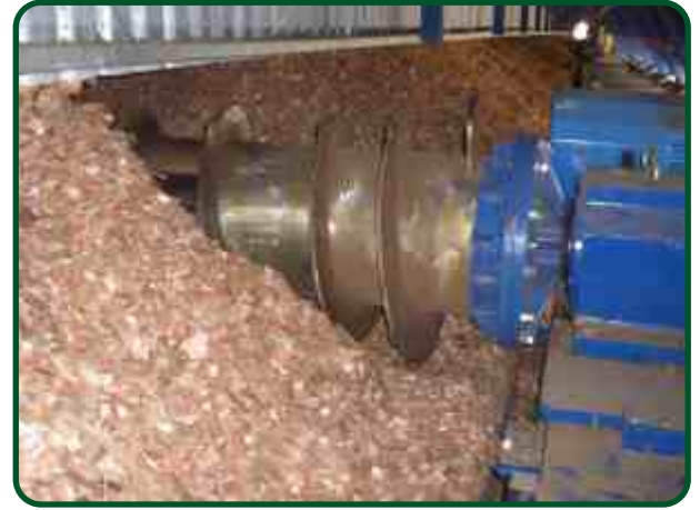
B iomass silo for 25.000m 3 loose storage capacity.
