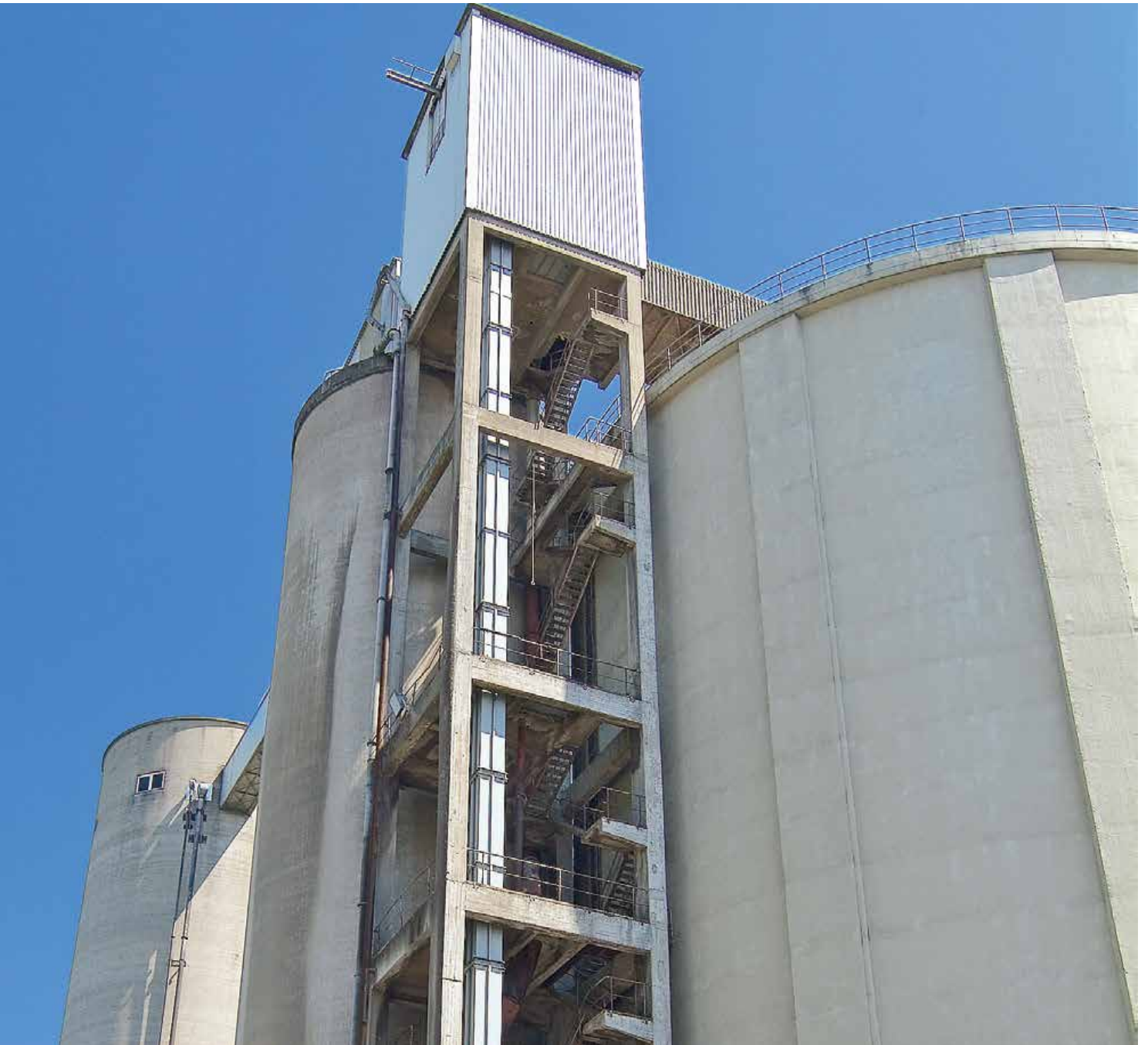
Bucket Elevator for cement silo feeding
