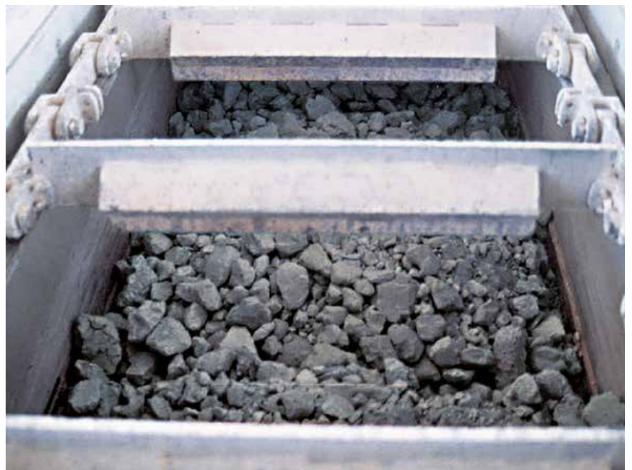
View into Chain Conveyor - Limestone feeding
