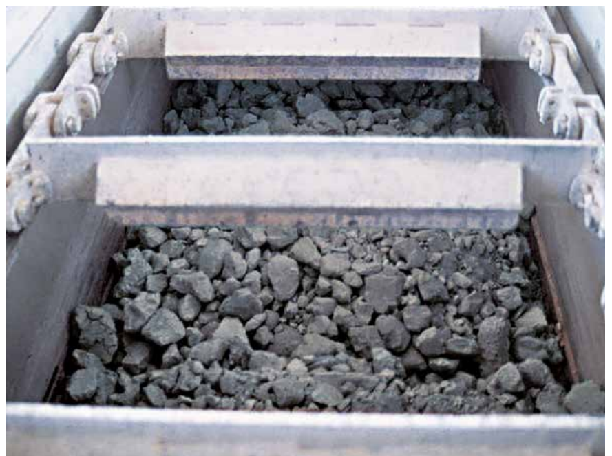
View into Chain Conveyor - Limestone feeding
