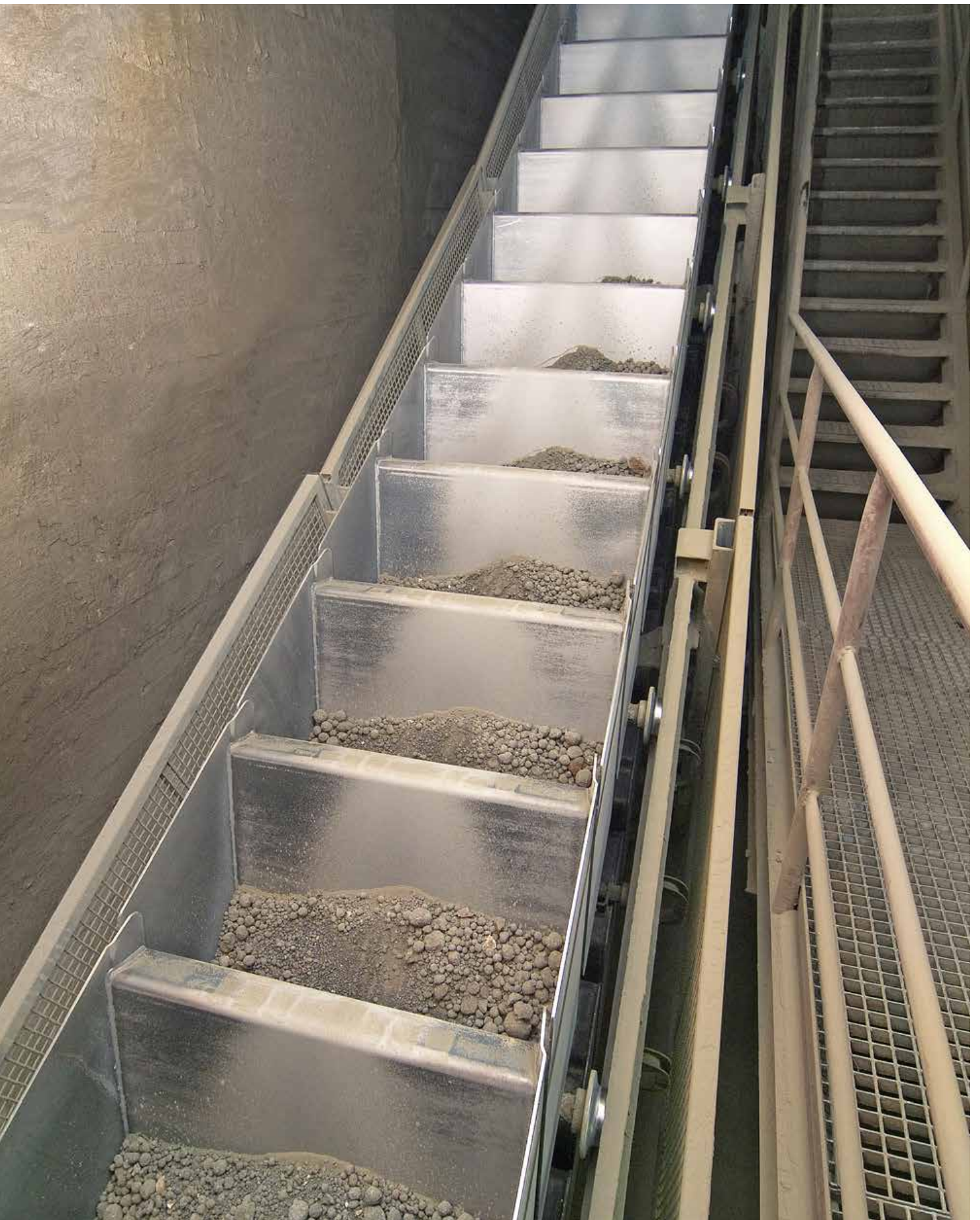
Clinker Transport with Conveyor type BZB
