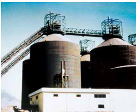
Steel silos, 30,000 t each
