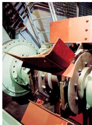
Scraper chain drive
