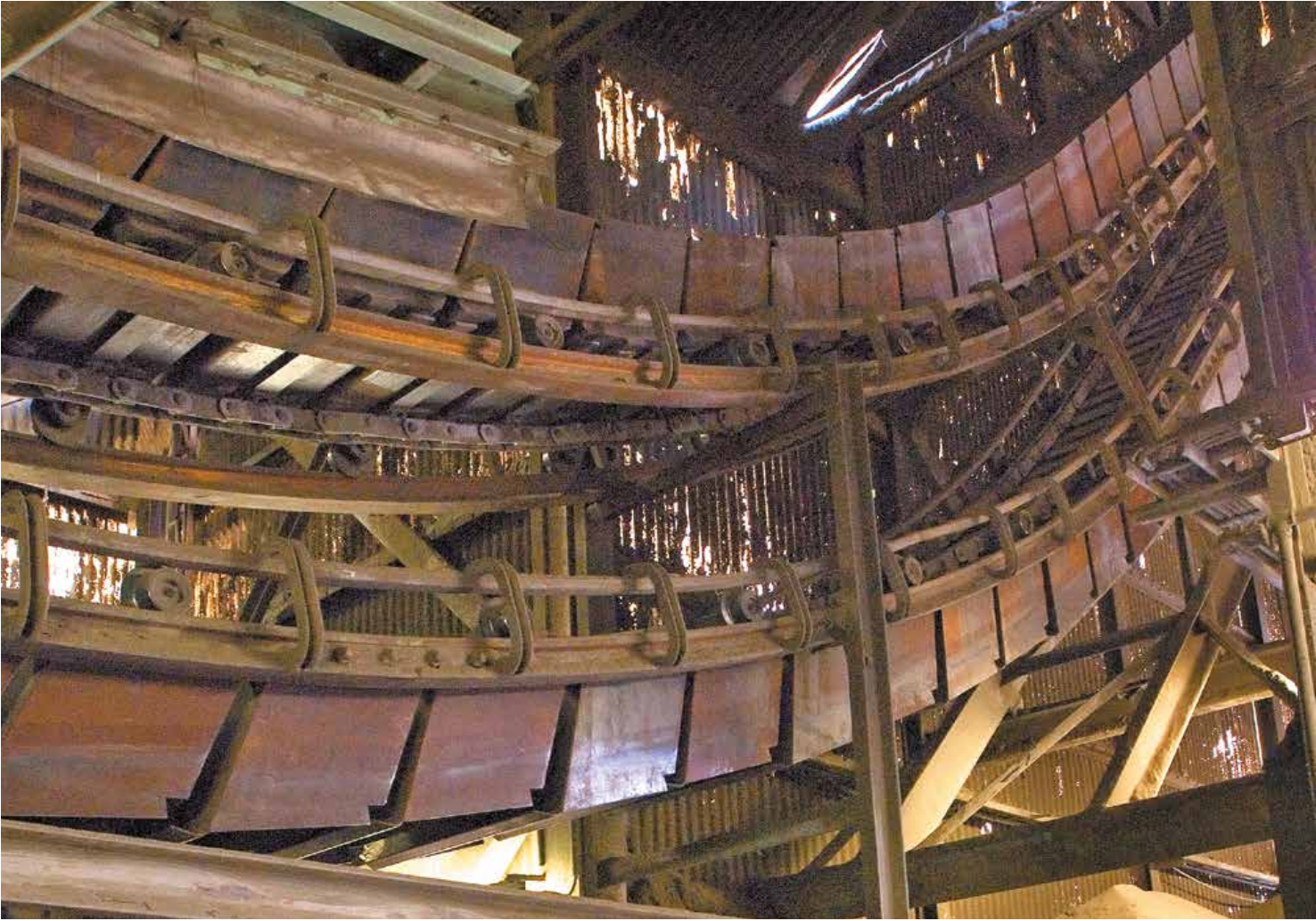
Bucket Apron Conveyor
