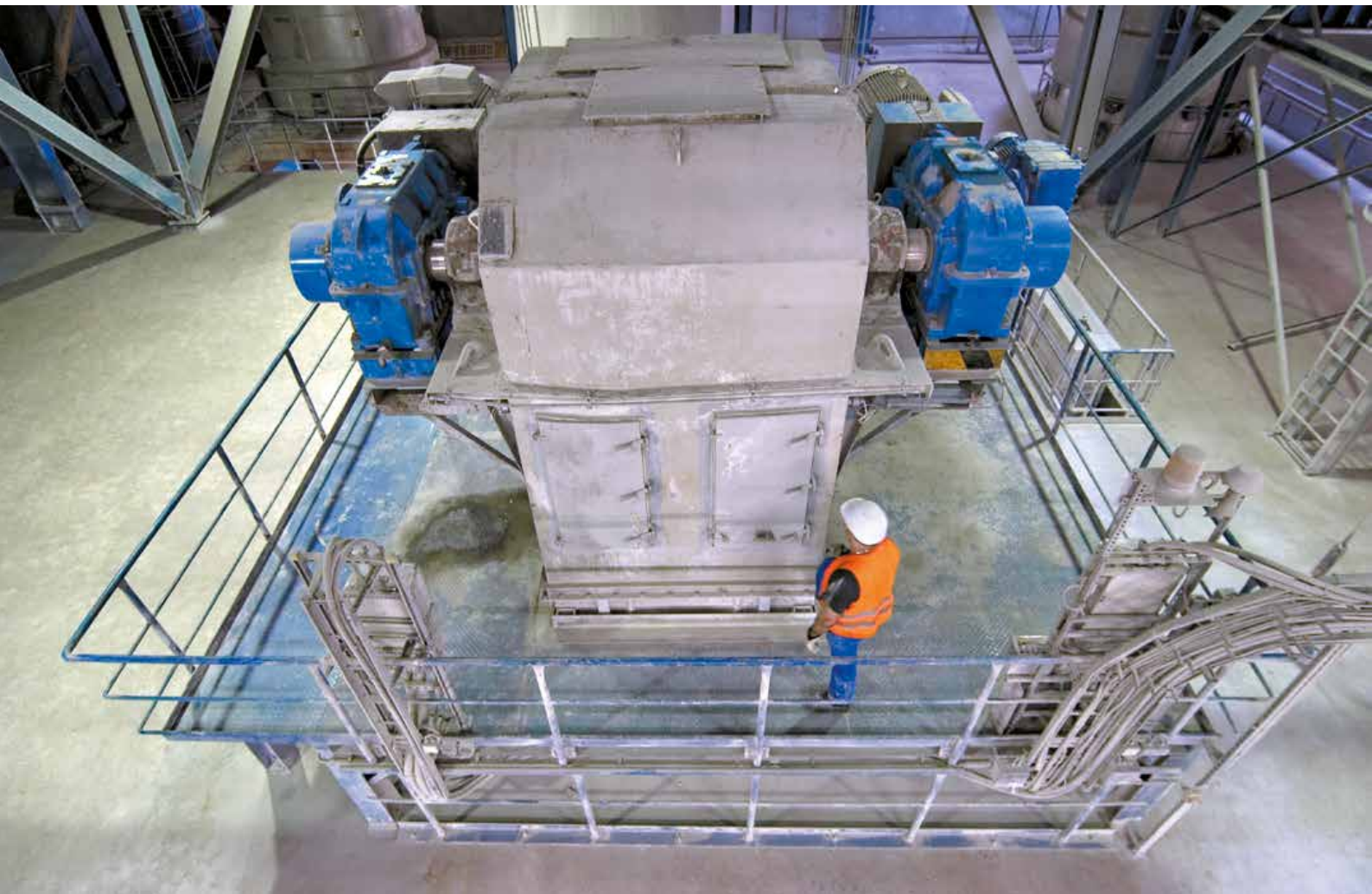
Head of Double Bucket Elevator
