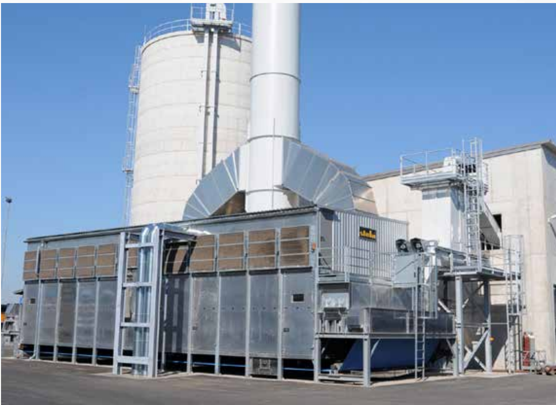
Project: Bioenergie Aschaffenburg Germany, Aschaffenburg Type: BT 1/6200-18 Year: 2009 Product: sawdust Dryer output capacity: 5,8 t/h from 50% - 10%
