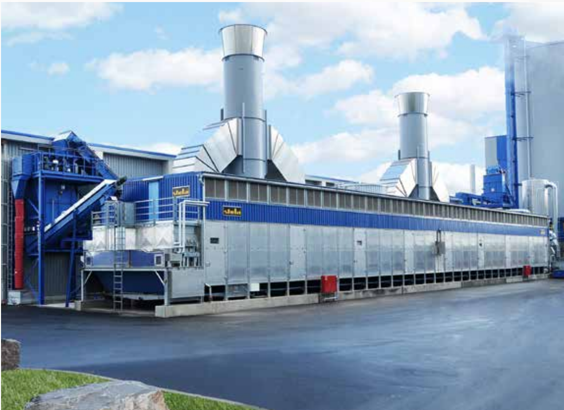
RWE Erndtebrück Germany, Erndtebrück Type: BT 1/6200-48 Year: 2010 Product: sawdust Dryer output capacity: 17,5 t/h from 50% - 10%
