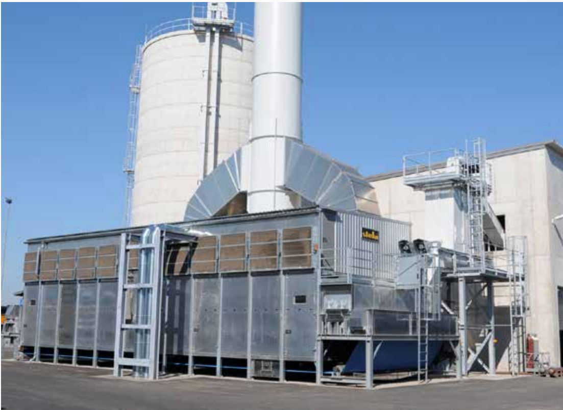
Project: Bioenergie Aschaffenburg Germany, Aschaffenburg Type: BT 1/6200-18 Year: 2009 Product: sawdust Dryer output capacity: 5,8 t/h from 50% - 10%
