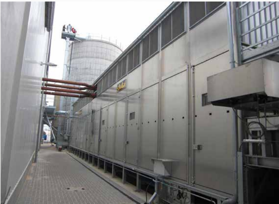
Project: BEN BioEnergie Germany, Buchholz Type: BT 1/6200-25,5 Year: 2008 Product: sawdust Dryer output capacity: 8,0 t/h from 48% - 8%
