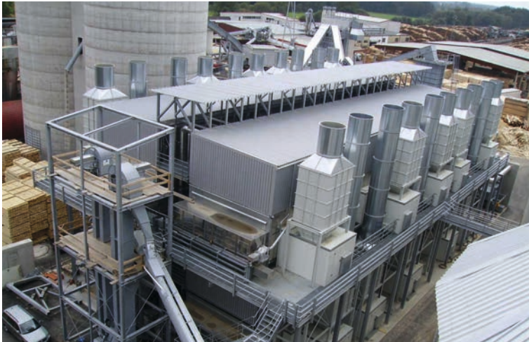
Project: Pfeifer Holz GmbH Germany Type: 4x BT 1/6200-36 Product: Sawdust
